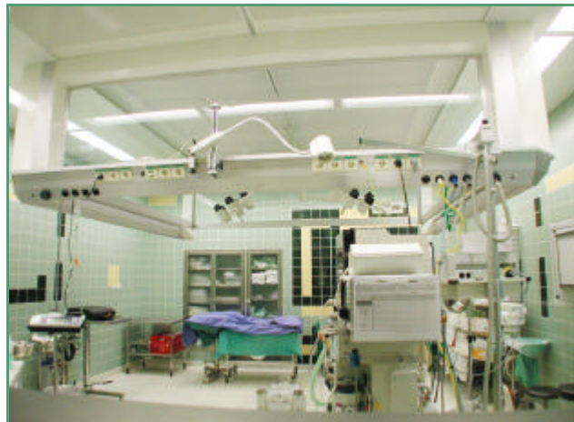
Operating theatre St. Josef in Moers, Germany, equipped with the ADMECO air conditioning ceiling ULA 26/26 UL-4 ECM, cabin model LFH 28/29, energy bridge MVB 45°/65° Typ U and ADMECO-Lux surgical lights model Typ 6SI/6SI.
